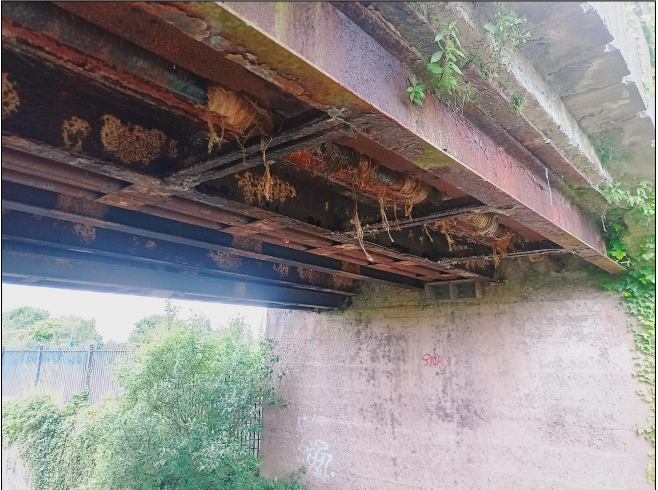
Figure 2. Heavily corroded steel structures in the bridge deck.
